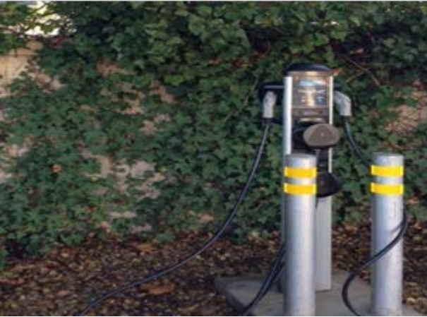
H Electric Vehicle Charging Station Infrastructure
