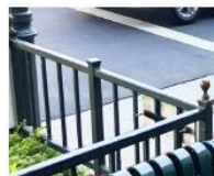
3 custom decorative green railing to match (e) streetscape Paint: Dunn Edwards DEA 180 Deep Pine
