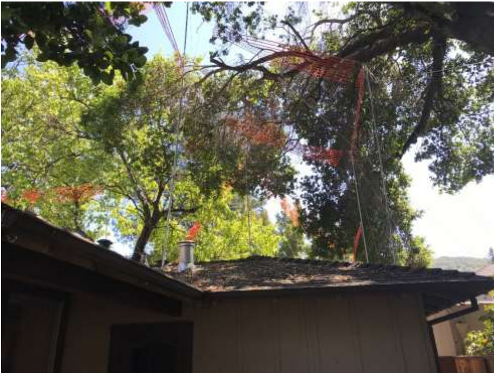
West side yard view looking South at the garage back wall, large Oak on the right.
